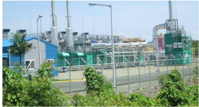
PIC's USAID-funded power plant, completed in June 2012. Caracol, Haiti © Gender Action 2013.
